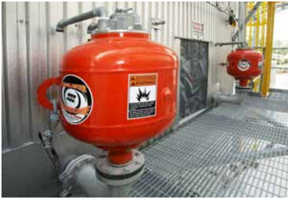
McGill's custom designed catalyst cleaning system reduces build-up and improves NOx reduction.
