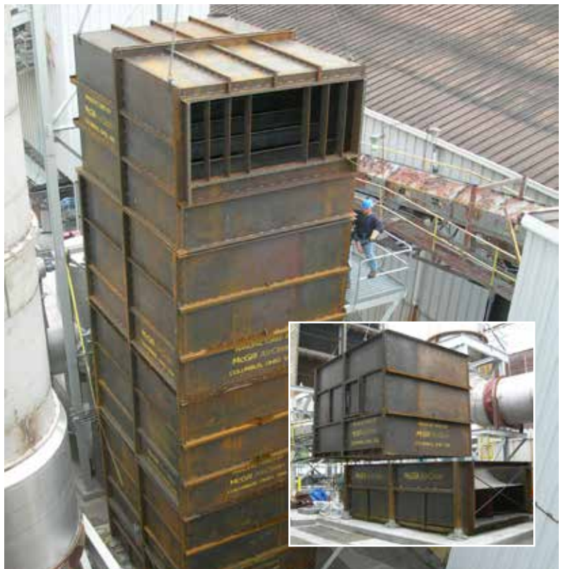
The top transition with flow distribution vanes is lifted into place, completing the erection of this three-module deNOx reactor. Inset: The modular design of the McGill deNOx reactor facilitates installation.
