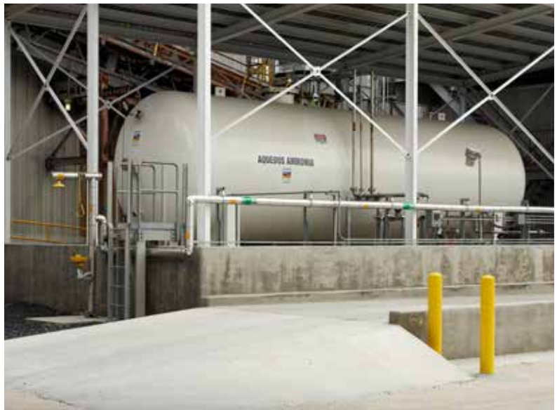
The reagent delivery system includes a storage tank, pumps, flow control valves, flow transmitter, and piping.
