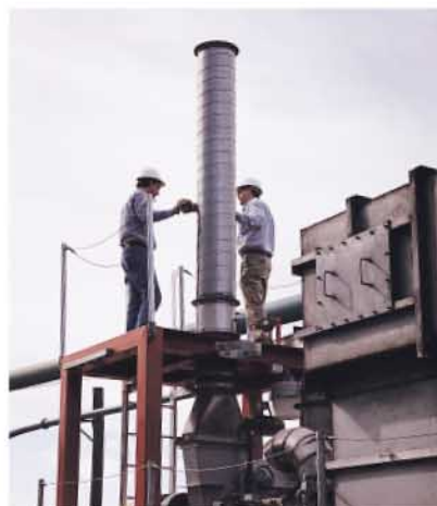
5. An exhaust stack is bolted into place on the mobile RTO platform.
