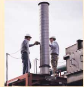
Removable exhaust stack with test ports is set up on site
