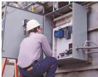
3. The RTO's burner management panel and electrical system is connected to your plant's power supply. Propane or natural gas supply is also hooked up.
