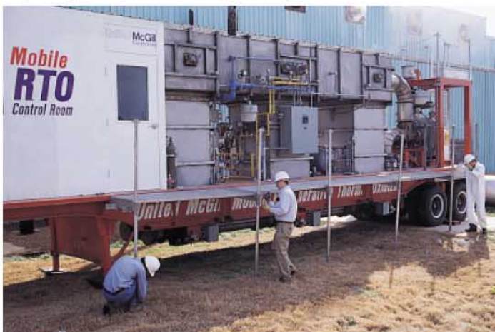
2. Walkways, stairs, and handrails are put into position to provide easy access to the RTO and its controls.
