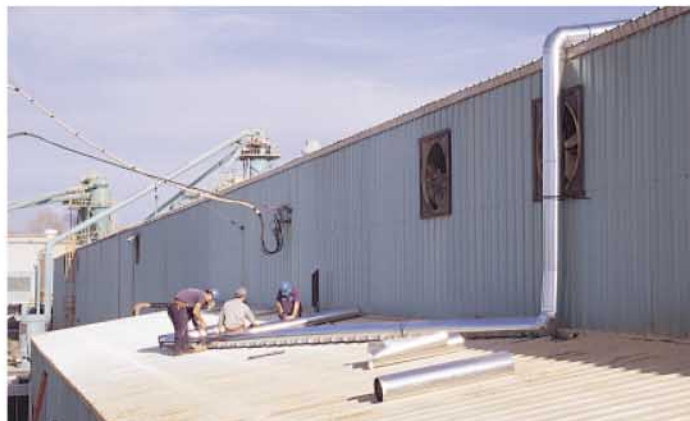
4. Ductwork is run from your process exhaust duct or stack to the RTO's inlet.
